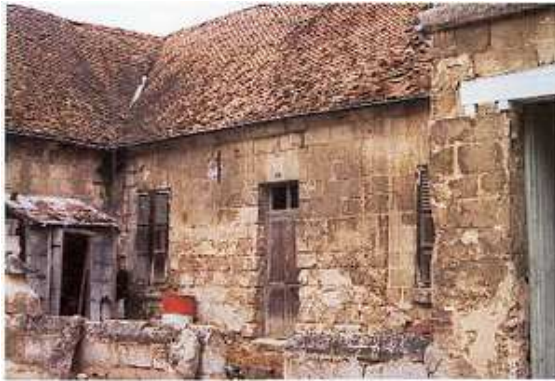
Saint-Just's house in 1989, at the time of its purchase. With its damaged roof, its gutted gable and the stones of its façade very degraded, it was in danger of destruction.
